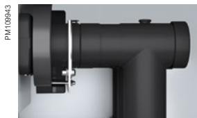
Current sensors around cable bushings
